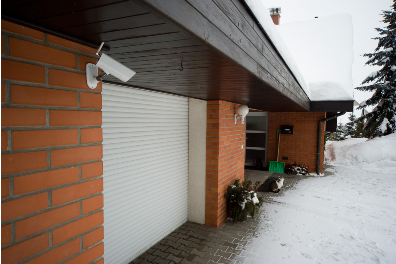
The EYE-02 placed under the roof near the car parking door. In this place the rain or snow can not reach the EYE-02.
